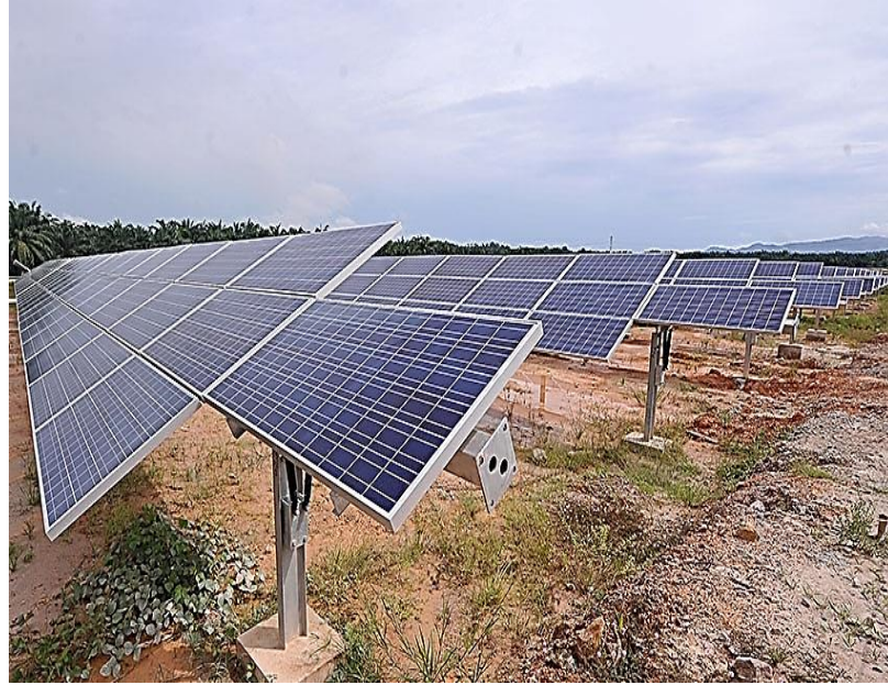
Figure 2.4 Solar power plant builds in Malaysia (Zaki, 2023)
