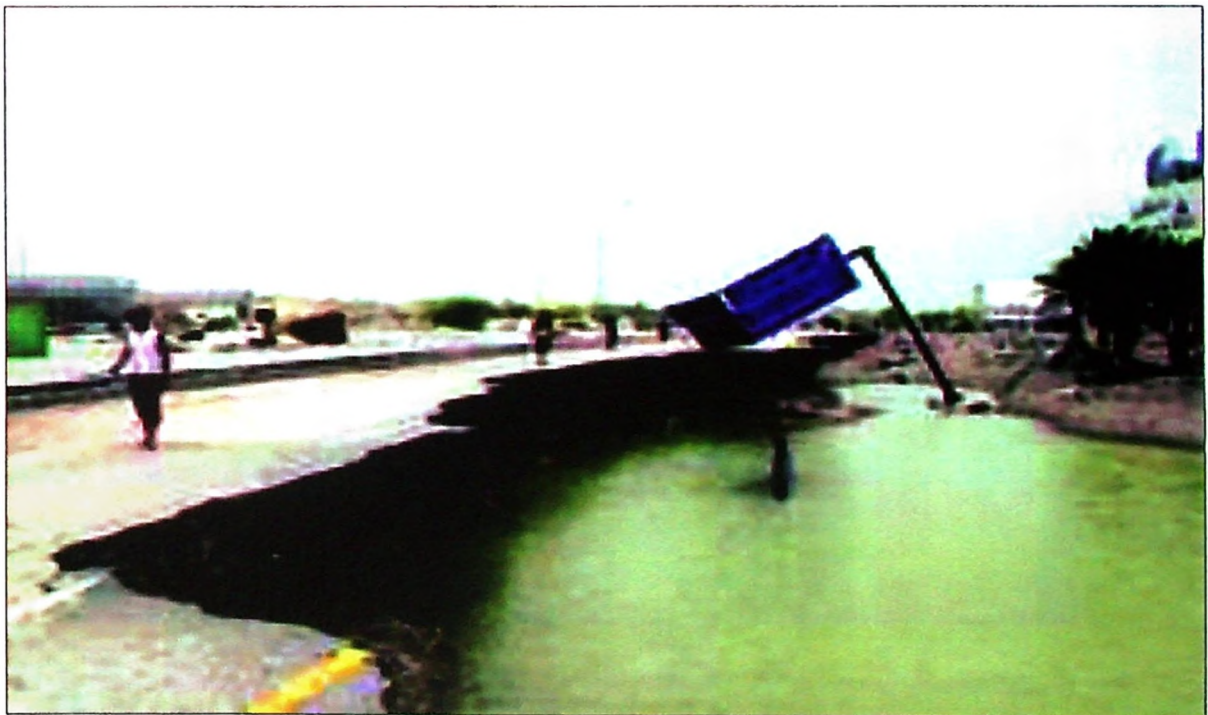
Figure 1.6: Damages in Oman's infrastructures caused by Cyclone Gonu (Roohoman, 2010)
