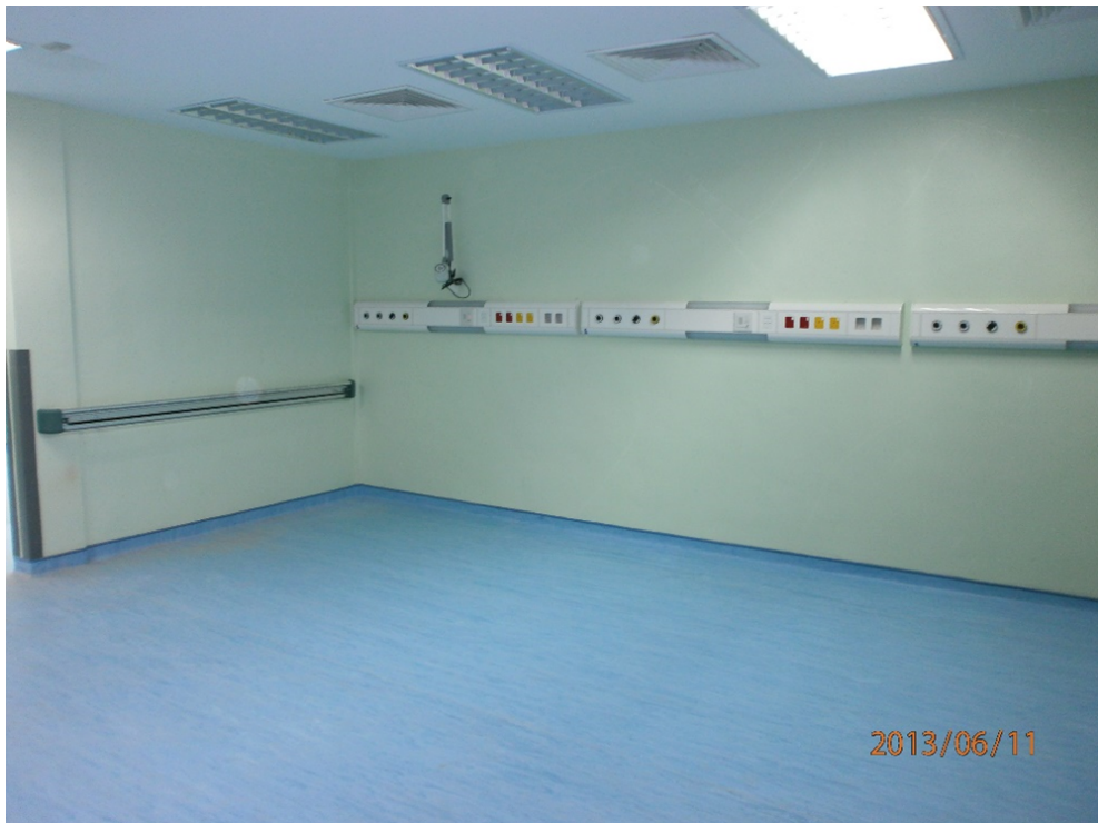
Plate 1.1 Lighting in a hospital ward.
