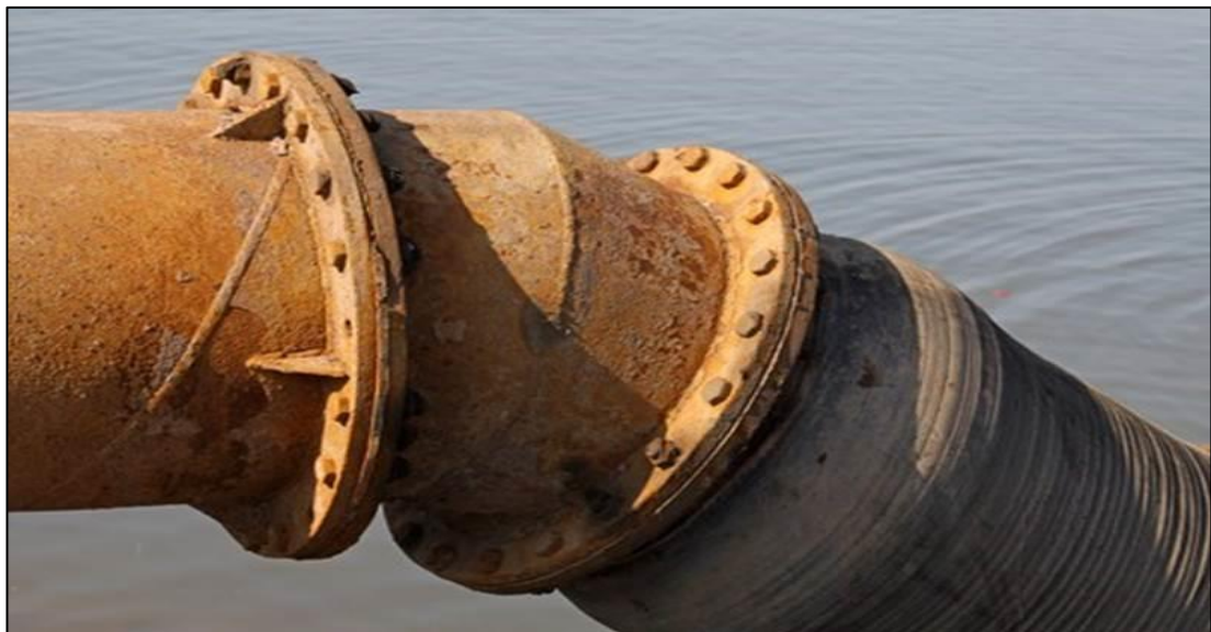
Figure 2. 3: Corrosion of carbon steel pipe (Kehr, 2018)
