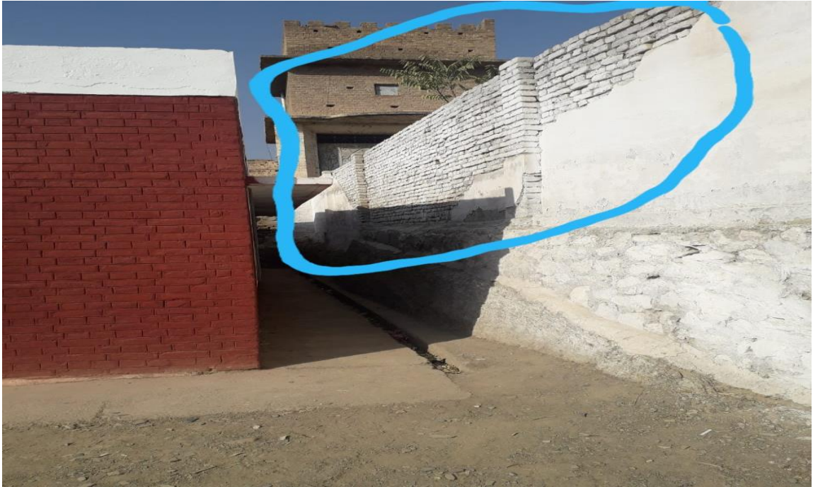
Figure 1.8 After an Explosion, the View of a Newly Constructed Boundary Wall of a Govt. Girls Primary School Ashraf Khel, Landi Kotal, Khyber Agency.
