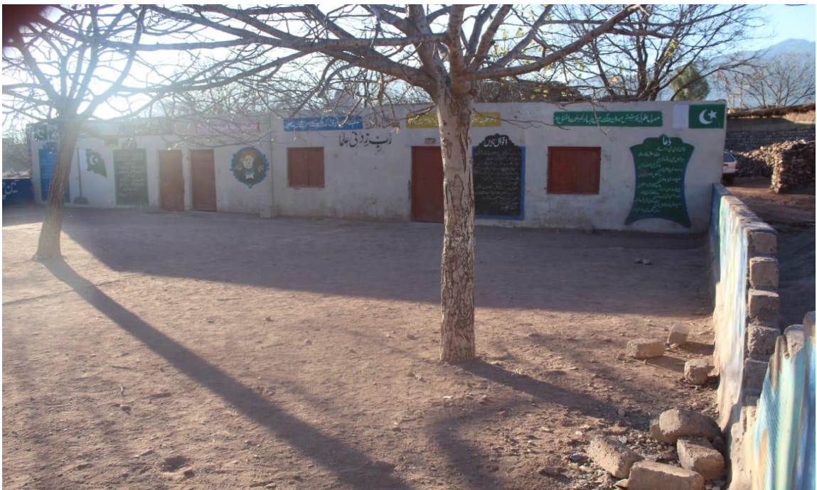
Figure 1.9 Terrorists Damaged the Wall of Govt. Boys Primary School, Malik Din Khel area, Tehsil Barra, District Khyber Agency, Pakistan
