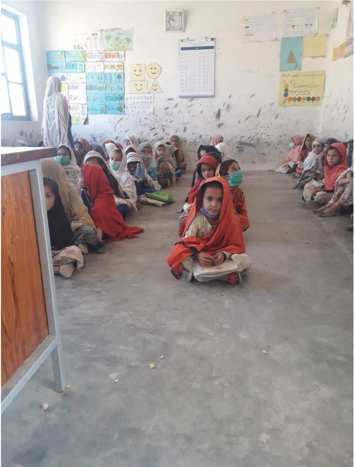
Figure 1.10 Dilapidated Condition of Government Girls Primary School, Sadu Khel Area, Landikotal, District Khyber Agency, Pakistan
