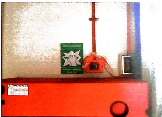
Figure A3.7: Picture of Fire Alarm
