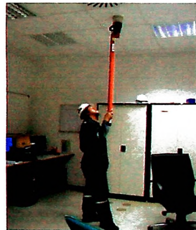
Figure A2.4: Picture of Testing for Smoke Detector
