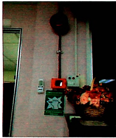
Figure A1.2: Picture of Fire Alarm
