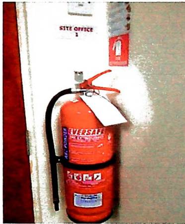
Figure A1.1: Picture of Fire Extinguisher
