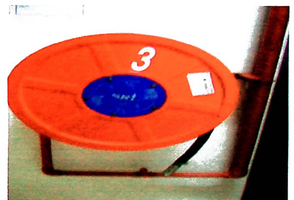
Figure A3.8: Picture of Hose Reel
