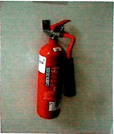
Figure A3.2: Picture of Fire Extinguisher
