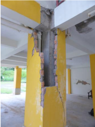
Cracking of the Masonry Wall Covering Column
