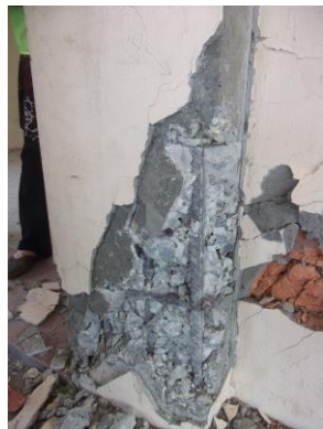
Cracking at the Bottom of Column
