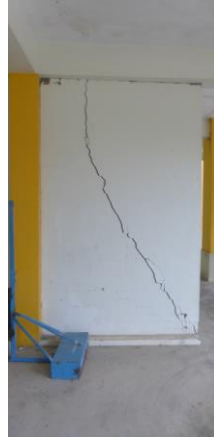
Diagonal Shear Crack on Masonry Infill Wall
