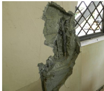
Beam-column Joint Damage
