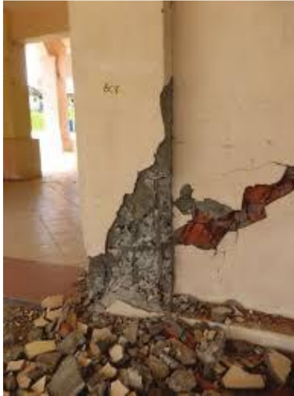
Figure 2.1: Structural Damage to the column of Hospital Ranau after Earthquake Event (Lim et al., 2017)
