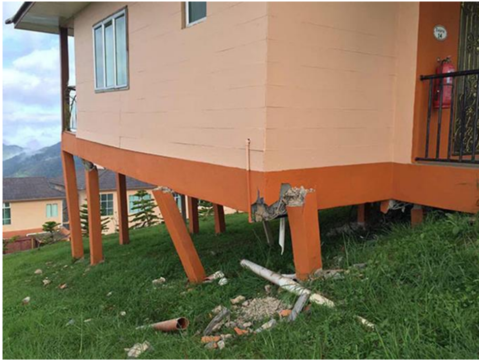
Figure 1.1: Damaged Stilts of a Motel in Ranau Due to Local Earthquake (Sario and Tan, 2015)
