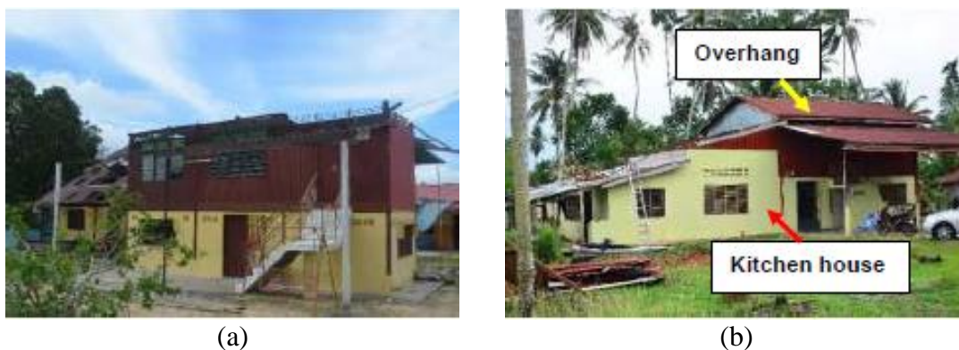
Figure 2.3 Failure of roof that initiate at overhang roof of rural house in (a) Balik Pulau, Penang and (b) Kepala Batas, Penang (Majid et al., 2016)
