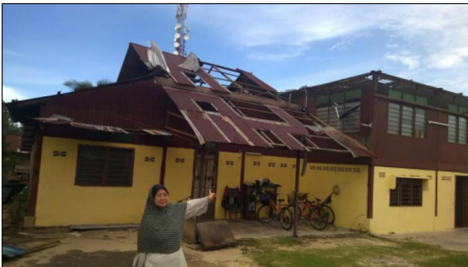
Figure 1.1 Roof damage during strong wind event
