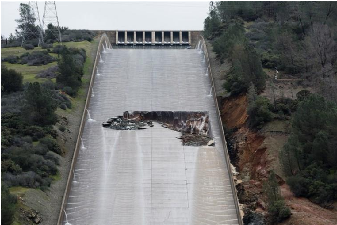
Figure 2.4 : The failure of Oroville dam's spillway (Patterson, 2018)
