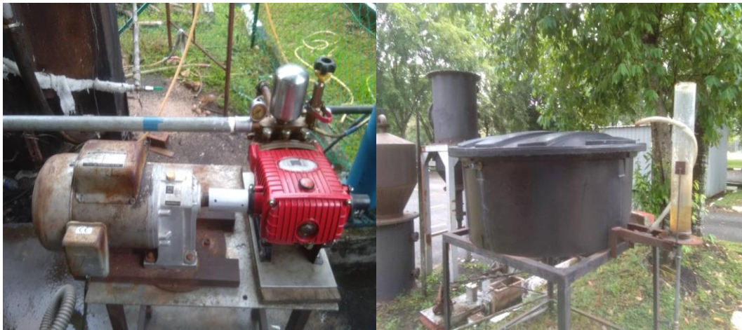
Figure 4.5: Water pump system with tank
