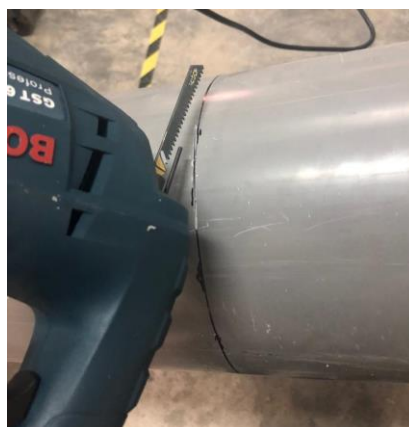
Figure 3.19: 50cm PVC pipe
