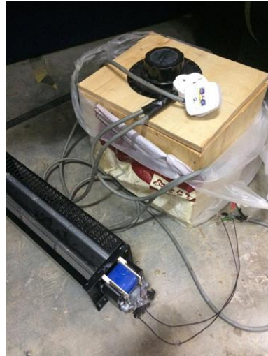
Figure 17: Transformer and roller fan
