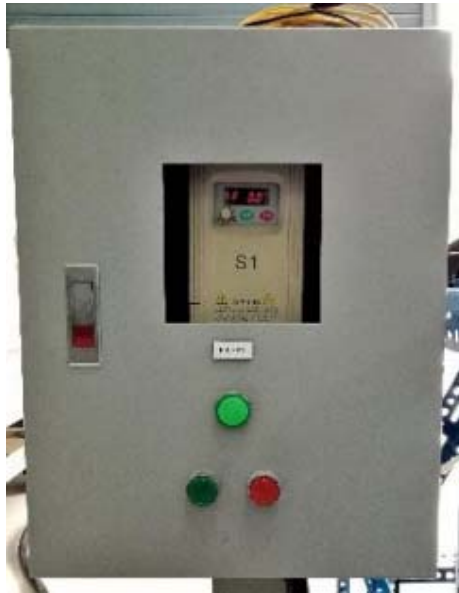
Figure 3.6 Motor speed controller unit
