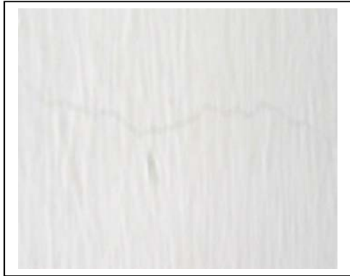
Figure 2.1(a): hairline crack
