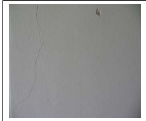
Figure 2.1(b): normal crack
