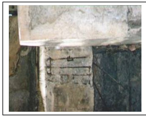
Figure 2.1(d): extreme width crack
