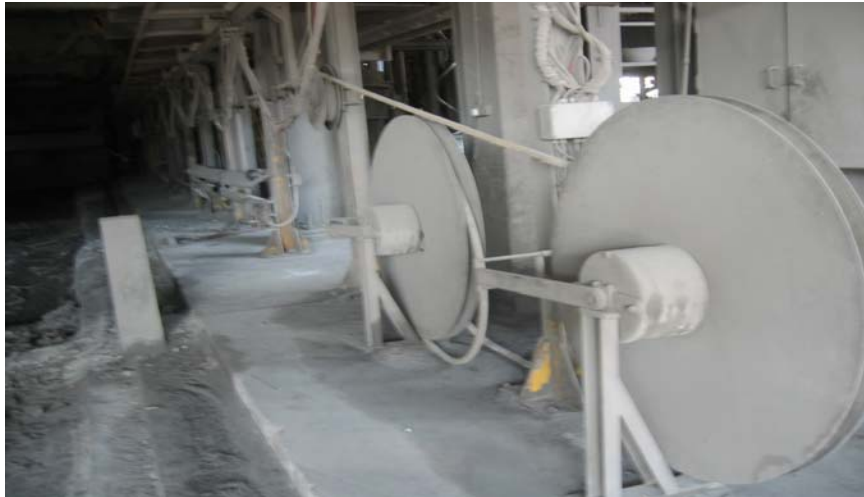
Figure 1.1 Rubber Pipe supply to Ladle Car
