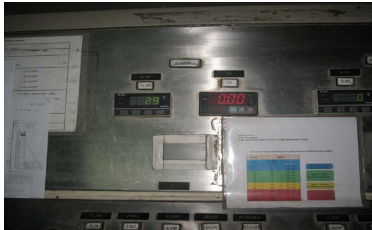
Figure 1.3 Control Desk of Existing System
