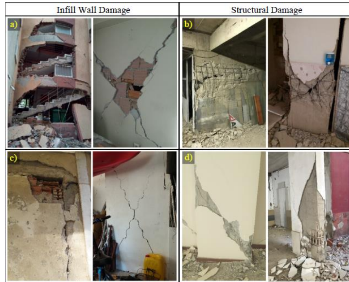
Figure 2.3: Structural and infill wall damage in Bayrakli, Turkey (Demirel et al., 2022)
