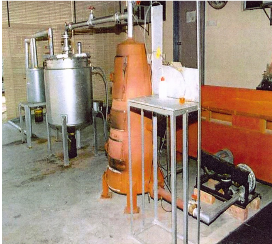
Figure 3.1: Overall view of the pilot plant for coal carbonization process
