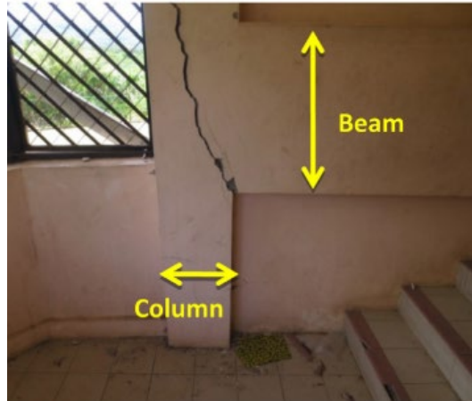
Figure 2.6: Damage of structure due to strong-beam weak-column effect (Alih and Vafaei, 2019)
