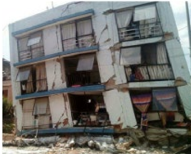
Figure 2.5: Collapse of the buildings in Mexico City (Jara et al., 2020)
