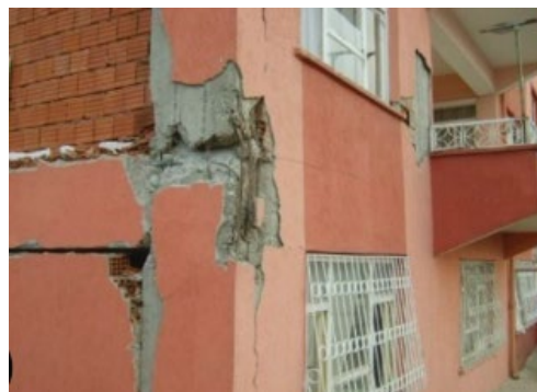
Figure 2.8: Damaged Structure Due to Inadequate Shear Reinforcement Spacing (Yon et al., 2018)
