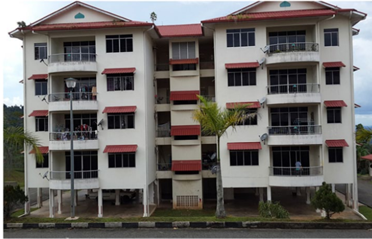
Figure 2.4: Typical weak first floor configuration for the RC buildings (Alih and Vafaei, 2019)
