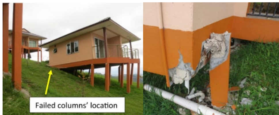
Figure 2.10: Failure of column on slope due to short column effect (Alih and Vafaei, 2019)
