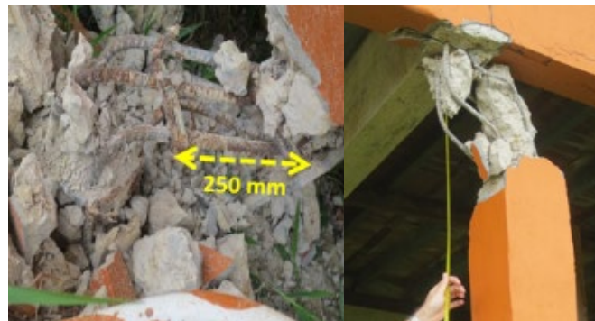
Figure 2.9: Damaged of columns due to large spacing between stirrups (Alih and Vafaei, 2019)
