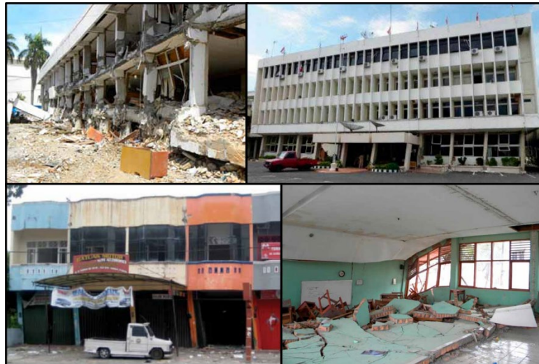
Figure 1.1: Damaged buildings in Padang City, Indonesia (EERI, 2009)
