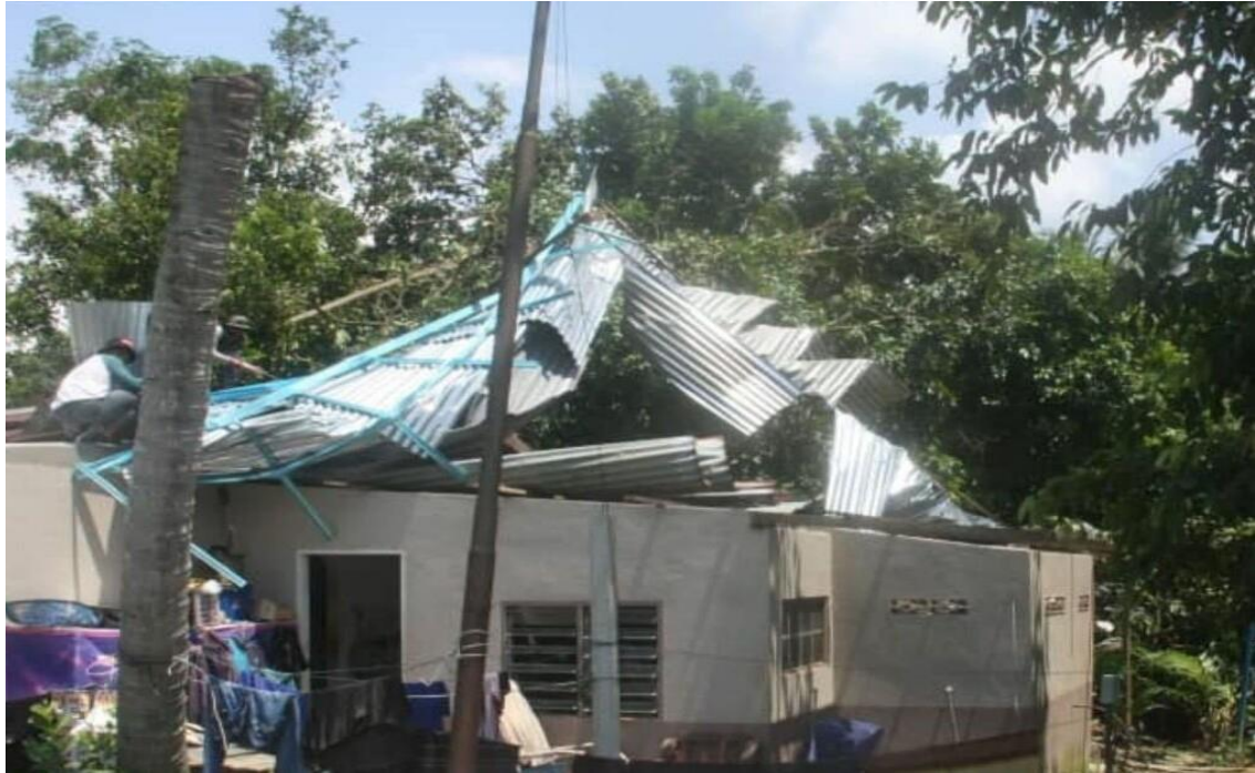
Figure 2.1 The roof damage in occurred in peninsular Malaysia
