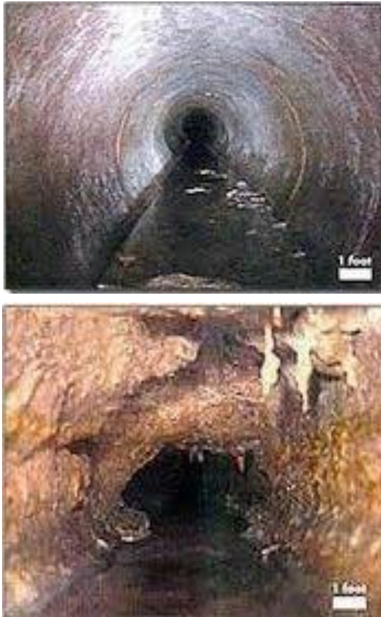
Figure 2.1 The sewer pipe before and after deposition of FOG. (Indah Water Konsortium, 2010)
