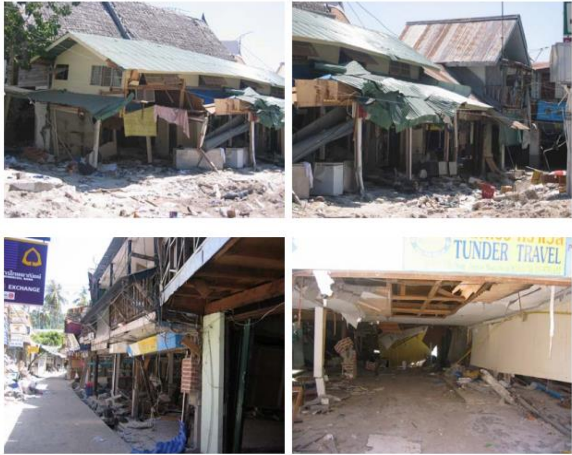
Figure 1.2 Damage to timber frame buildings in Phi Phi Island, Thailand (Saatcioglu et al., 2005)
