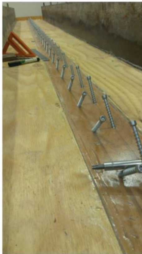
Figure 2.4: Fully threaded screws fitted at \pm 45^\circ on timber joist (Sebastian, et al., 2016)
