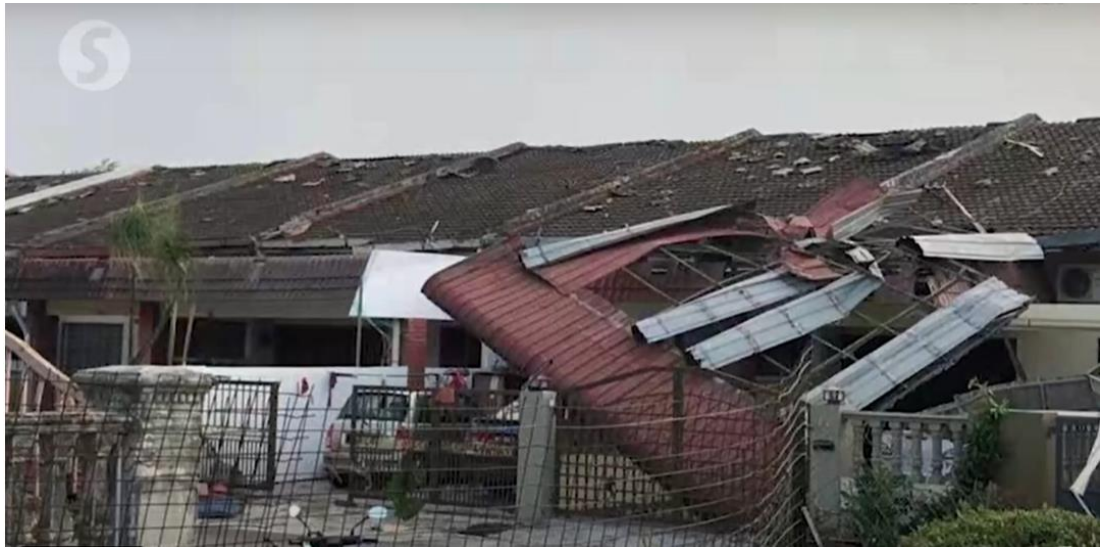
Figure 1.1 Roof damage as reported by The Star, 30 th Jan 2022
