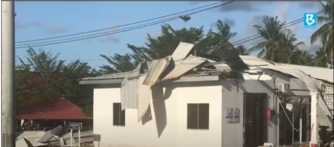
Figure 2.1 Roof damage as reported by Bernama, 26 th March 2021
