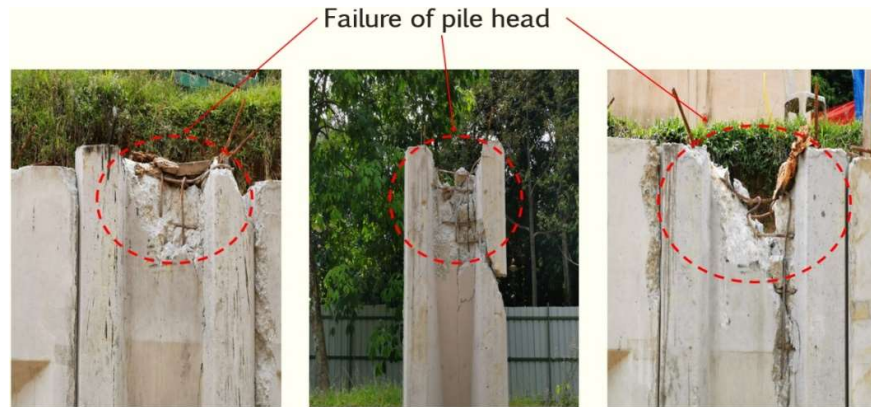
Figure 1.13: Failure of pile head
