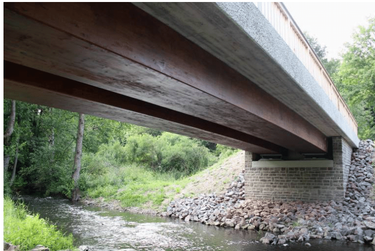
Figure 2.2 (a): TCC bridge "Birkbergbrücke" in Germany (Photo adopted by Jens Müller, n.d)
