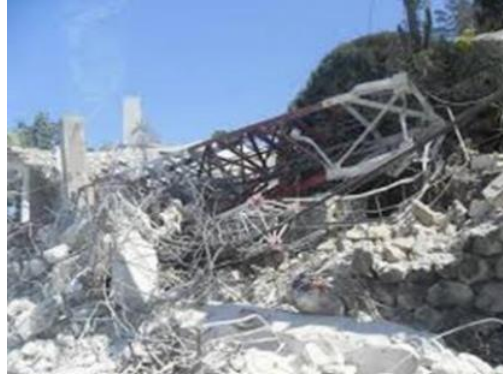
Figure 2.1: Damaged Communication Infrastructures (Bendimerad, 2013)
