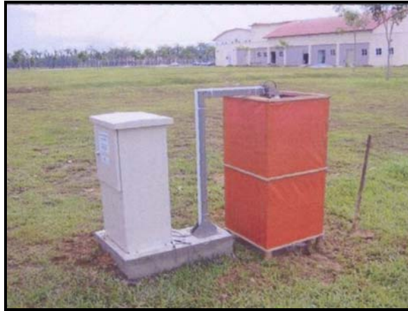
Figure 3.4: ISCO 4110 Ultrasonic Water Level Logger
