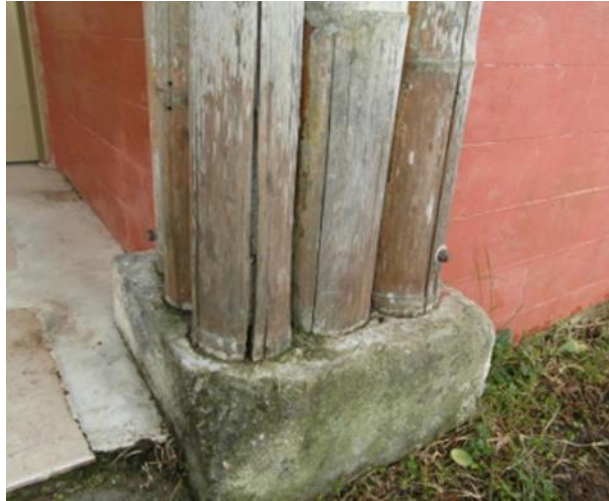
Figure 2. 6 Fungal damage due to exposure to sun and rain (Kaminski et al., 2016)
