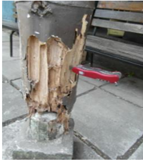
Figure 2. 5 Severe external damage from termite attack (Kaminski et al., 2016)
