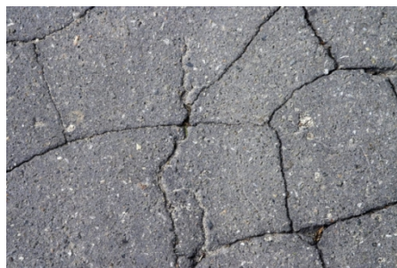
Figure 2.1: Common Fatigue Cracking Occur on Road Surface
