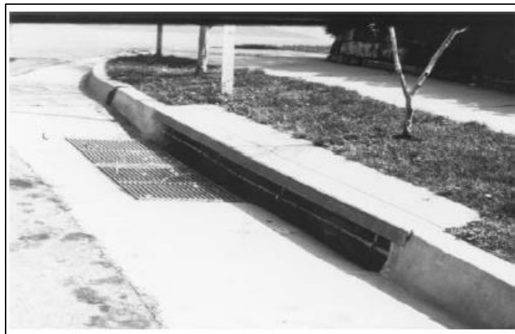
Figure 2.4 Sweeper Combination Inlet. (DID, 2012)
