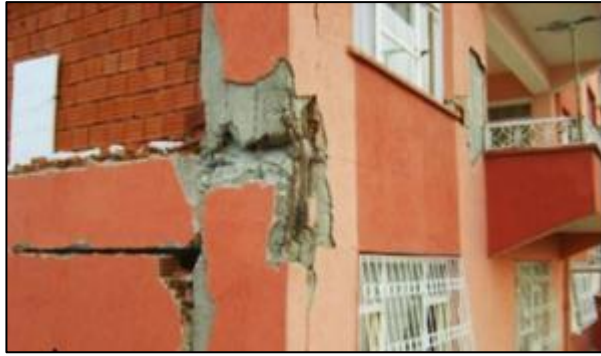
Figure 2.4: Damaged Structure Due to Inadequate Shear Reinforcements Spacing (Yön et al., 2017)
