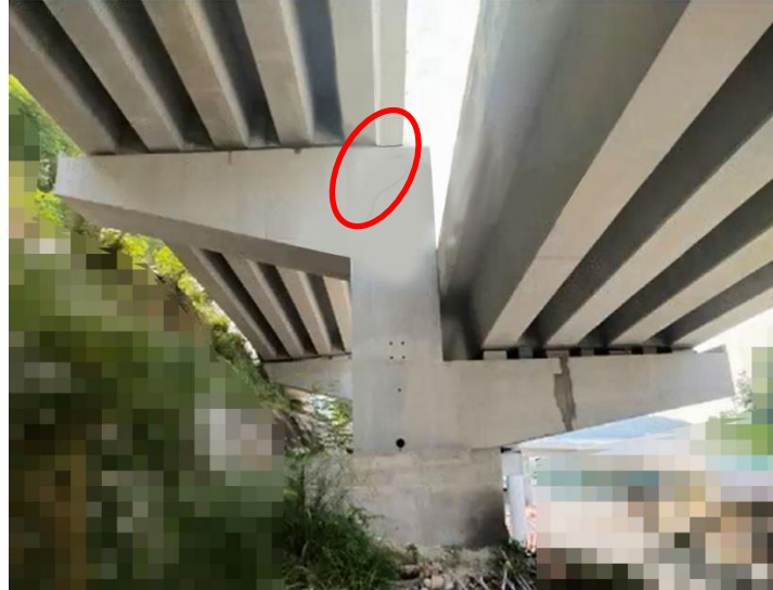
Figure 1.4: Staggered Crossbeam Pier with Cracking Problem (Red circle mark the cracking position)
