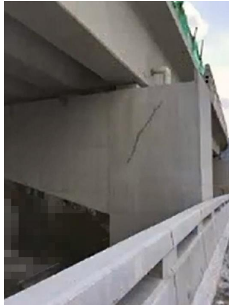
Figure 1.5: Staggered Crossbeam Pier with Cracking Problem (View from Middle Bridge Deck)
