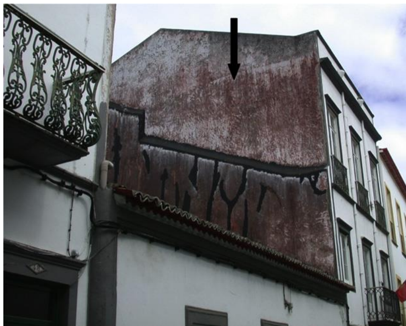
Figure 2.1 Wall covered in dark red growth (arrowed) of Trentepohliales. This algae is the primary colonizer in Singapore (Gaylarde, et al., 2011).
