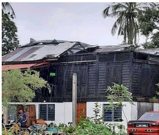
Figure 1.1 Roof damage during windstorm event
