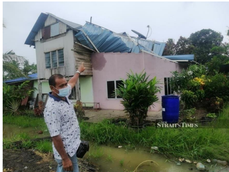
Figure 1.2 Roof damage in Indera Mahkota Dua, Kuantan (New straight times, 30 October)
