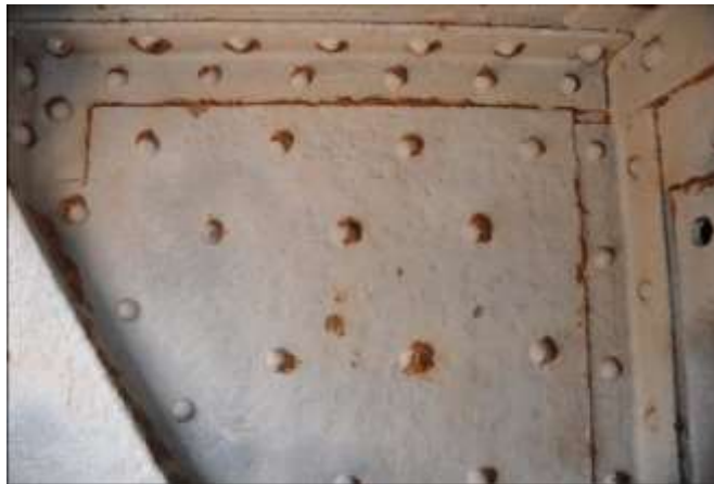
Figure 2.5 example of pitting corrosion of a steel plate. (Markova, 2016)
