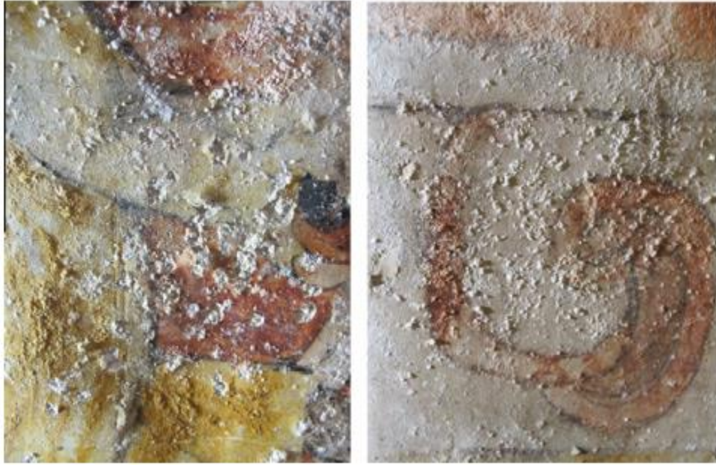
Figure 2.7 Salt efflorescence on surfaces of mural paintings and detachment of the paint layer (Chelazzi, et al., 2013)
