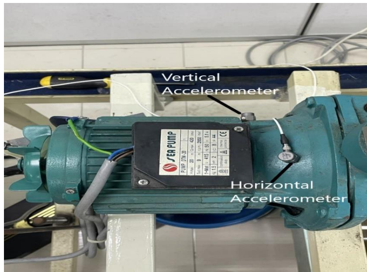
Figure 3.5: The position of the accelerometer attached to the centrifugal pump
