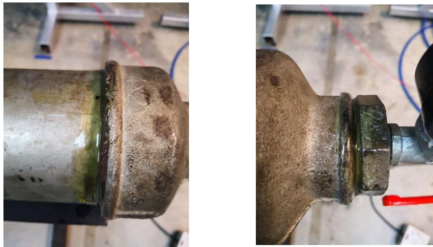
Figure 3.4: Gas leakages is solve using epoxy resin
