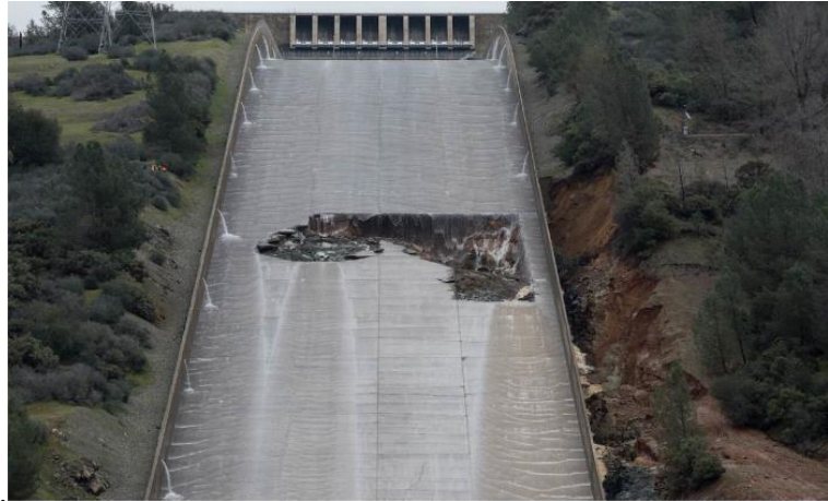
Figure 2-2: Cavitation damage occurred on the Oroville spillway surface
