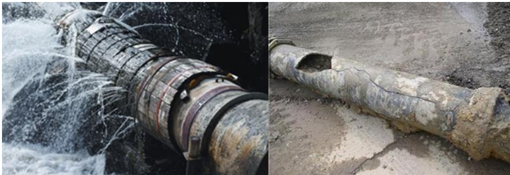
Figure 1.3: Pipes broken from water hammer
