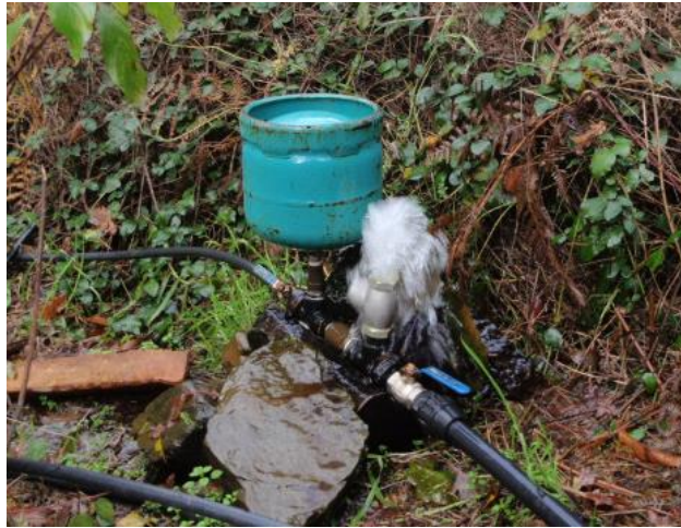
Figure 1.1: Hydraulic ram pump used in rural area
