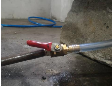
Figure 3.14: Valve controlling fuel flow
