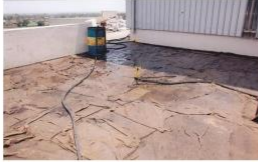
Figure 2.4: Water sprinkler and absorptive material [24]
