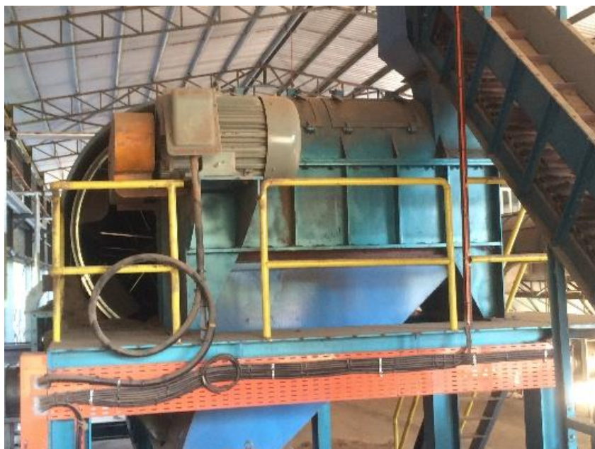
Figure 1.5 Hammer Mill to shred EFB
