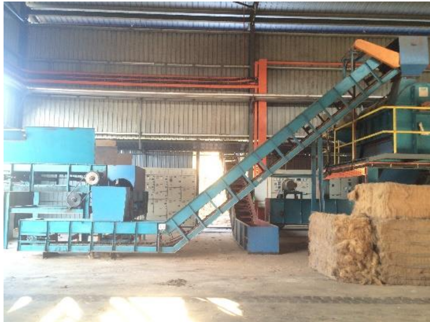
Figure 1.4 Feeding conveyor to hammer mill
