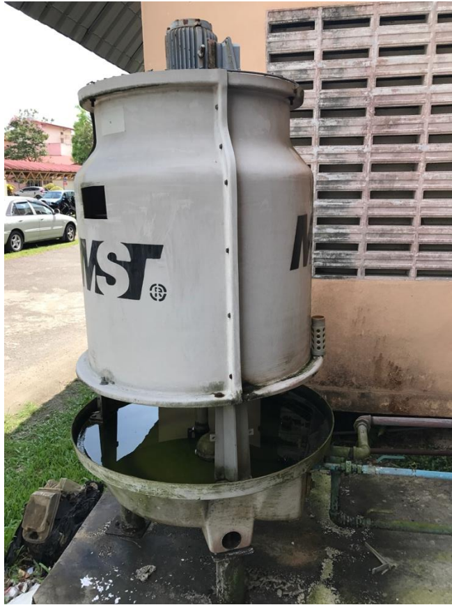
Figure 3.9: Cooling Tower placed outside engine lab
