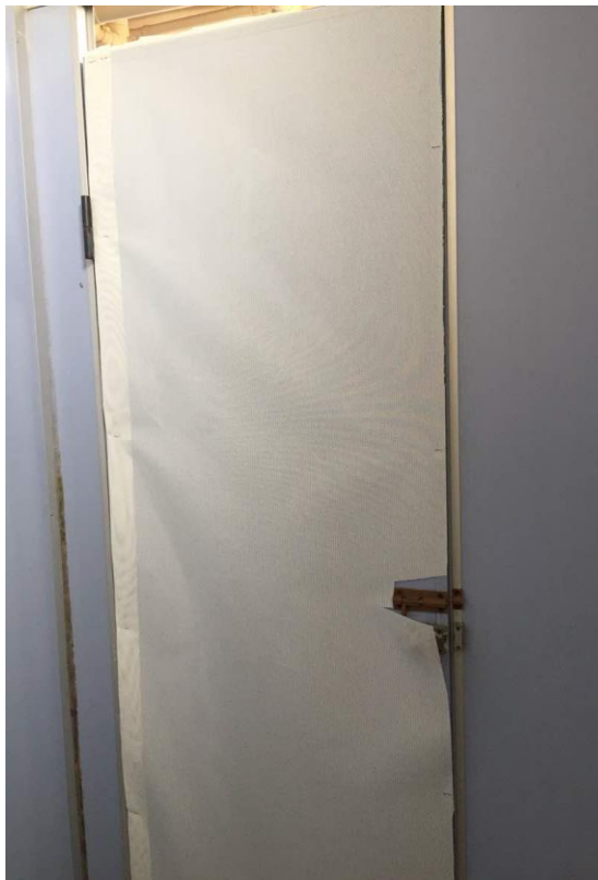
Figure 3-7 : Deodoratex application in vertical conditions at toilet and shower doors using Deodoratex Type 03
