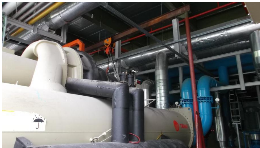
Figure 1.2: The side view of a chiller machine.
