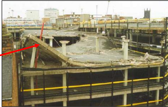
Figure 1.3 Collapse of Pipers Row Car Park, Wolverhampton (Wood, 1997)
