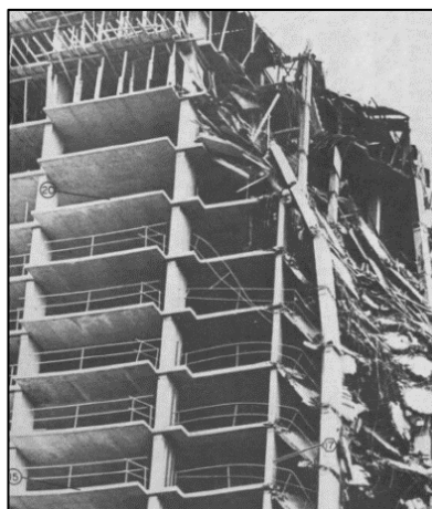
Figure 1.4 View of the failure zone of Skyline Plaza (Leyendecker and Fattal, 1977)
